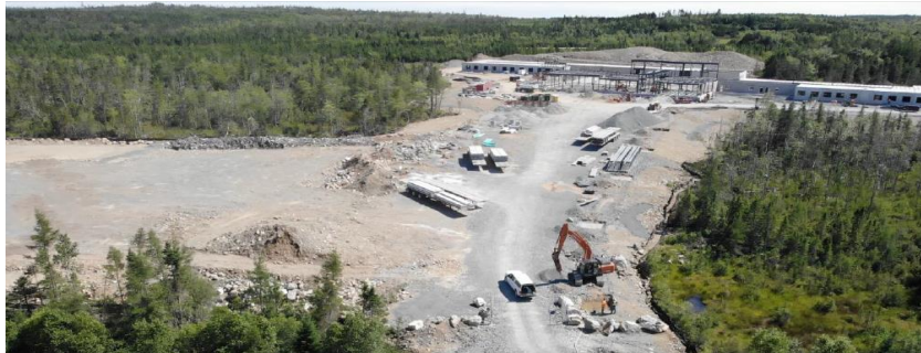
Aerial photo from the north, looking towards the main entrance. Sports field on left side.
